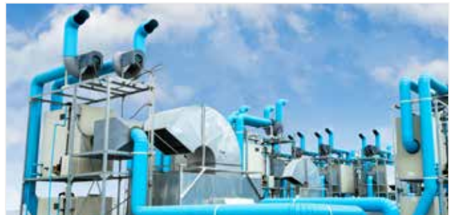
Air Exchanging and Filtering
