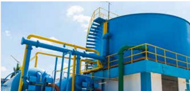
Water Treatment Pumps
